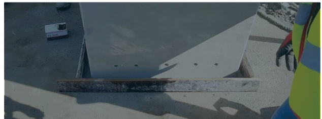
Reinforcement continuity detail from monolithic raft to precast column, with rigid joint executed by mortar injection into reinforcement ducts
